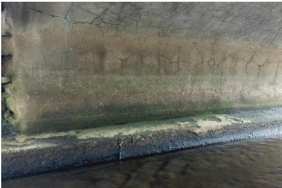
Figure 5.6: Cracking of Bridge Soffit Repairs
