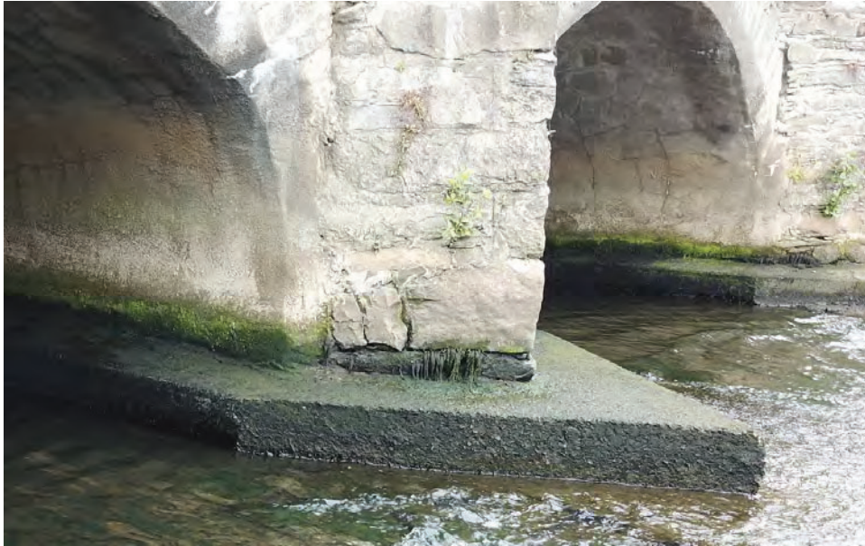
Figure 5.7: Masonry Joint Defects
