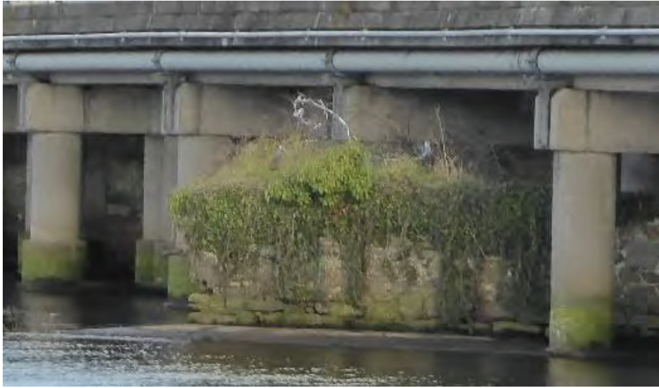
Figure 5.5: Vegetation Growing on Arklow Bridge
